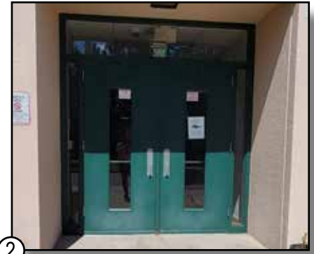
2 HOLLOW METAL DOORS & HOLLOW METAL STOREFRONT
