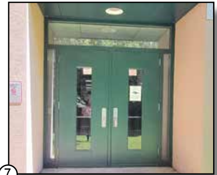
7 HOLLOW METAL DOORS & HOLLOW METAL STOREFRONT
